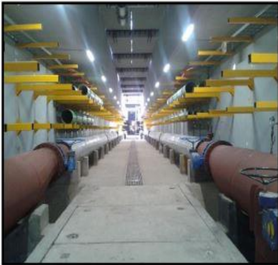
GIFT Utility Duct: Gandhinagar
